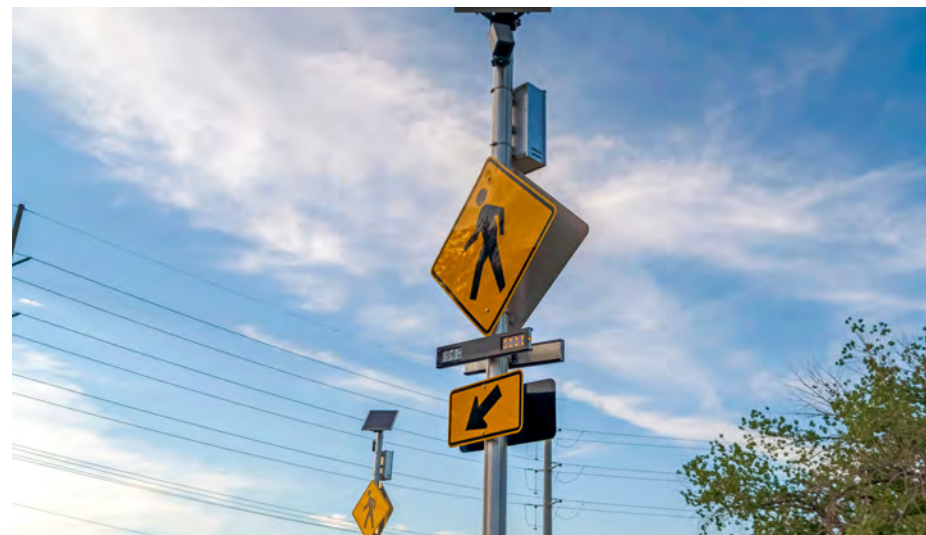
FIGURE 13. RECTANGULAR RAPID FLASHING BEACON (RRFB)
